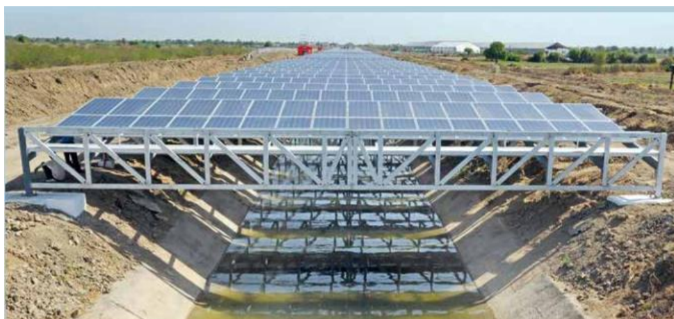
Figure 2-4 Canal top Solar PV system in Gujarat
