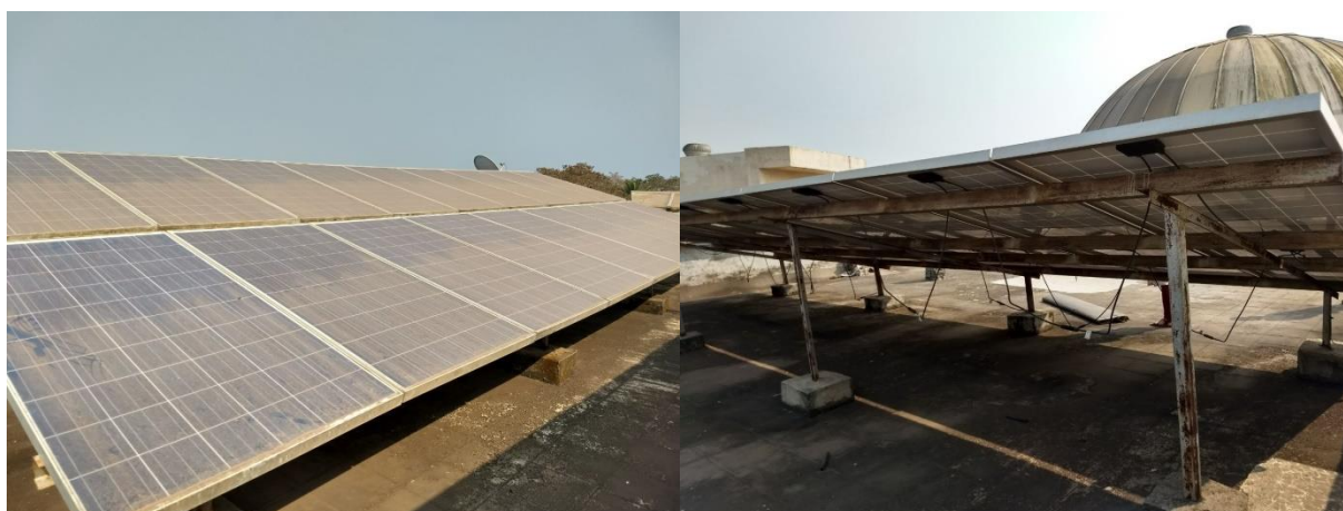
Figure 4-4 Study of existing solar PV installation at Pt. Deendayal Upadhyay Bhavan, Porvorim
